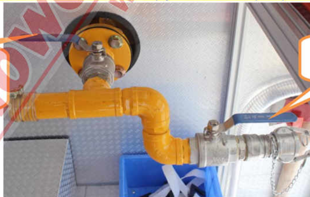
Foam Outlet Valve (Control foam in tank and fire)
